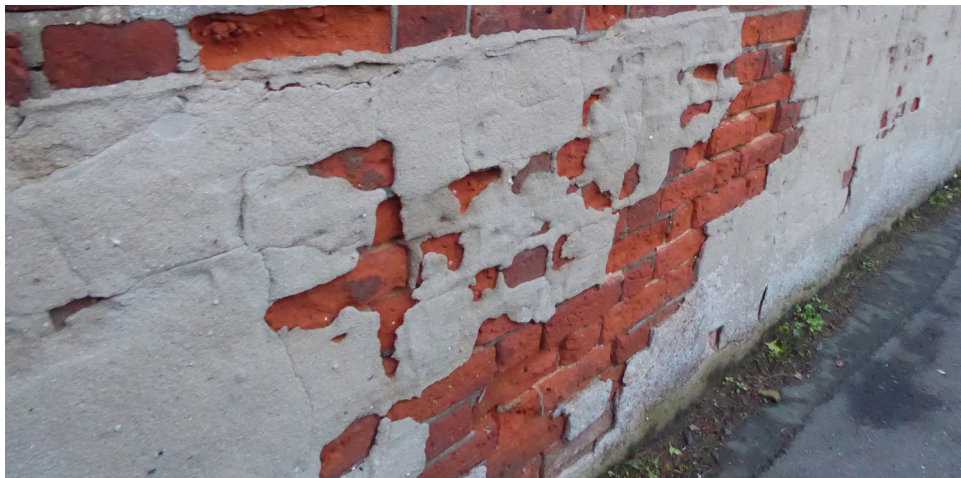
Figure 45 Peeling cement render from the boundary wall to the Old Rectory
