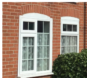
Figure 40 Loss of original features with the replacement of timber sashes and casement with uPVC
